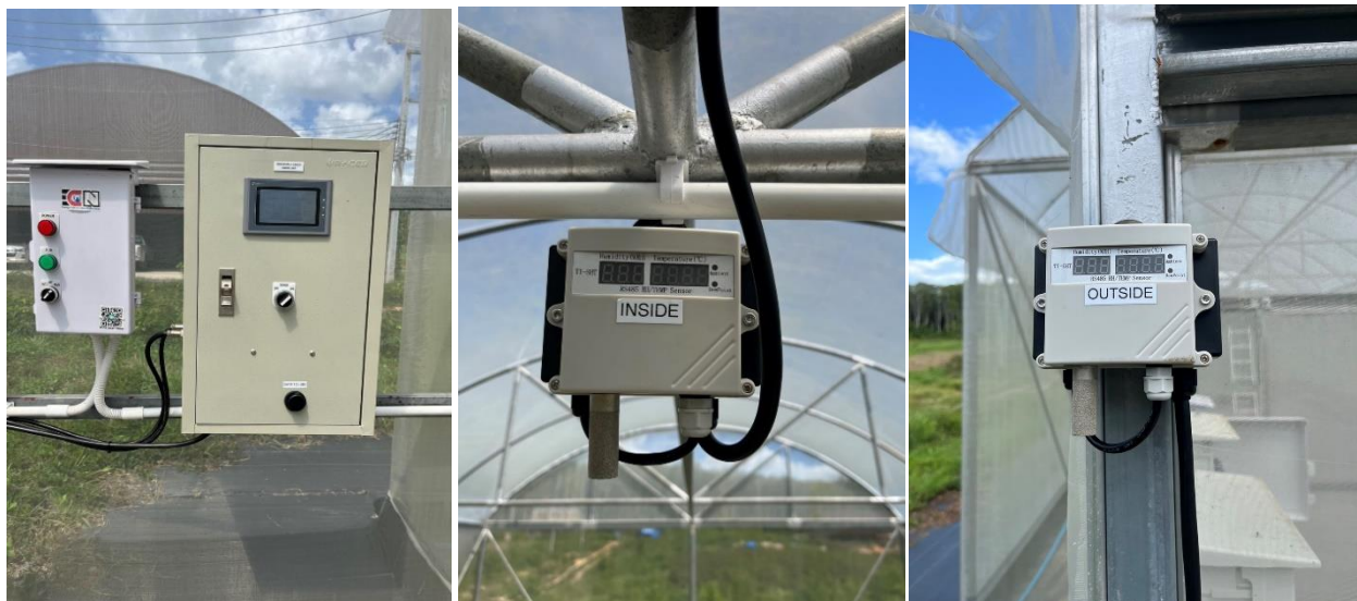
Figure 2 Ventilation control, Temperature and Humidity sensor
